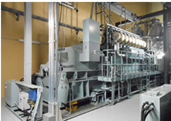
Gas engine powered CGS
