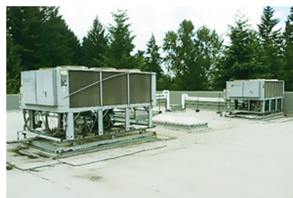
Air conditioning system installed on the roof
