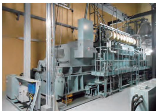
Gas engine CGS
