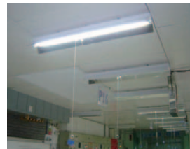
Fluorescent lamps with pull-switches for independent control
