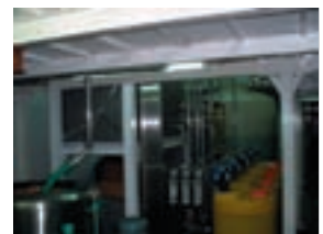
Sedimentation treatment tank at an ink plant in China
