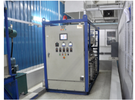
Jointly-developed liquid waste treatment system
