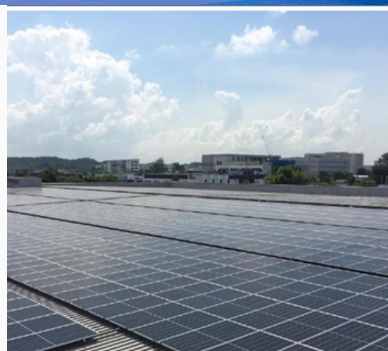
Rooftop solar panels at Singapore Epson Industrial
